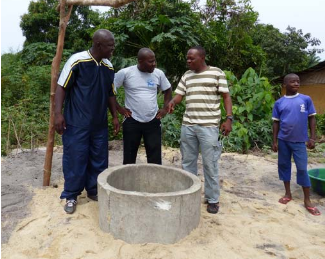
Figure 1. Construction of the water pump underway in Samuel Brown town in Liberia (Photo: Manjula Tiwari).
